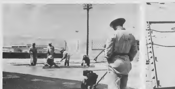
LAGO WORKMEN assigned to the Lago Sport Park project are shown assembling screeds, or the lengths of board which are set at the desired height and then used as guides to level the concrete as it is poured.
